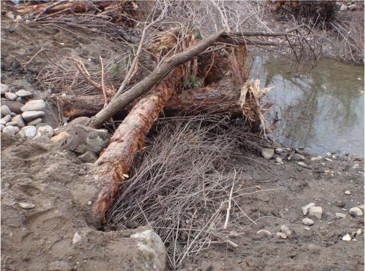
Figure 1. Wood structure at Lower Seiad Pond showing two criss crossed pines (we prefer Douglas fir for longevity), fine brush pinned beneath, and a live willow saved from the excavation on top (willow was chopped up by beaver to make a dam in Seiad Creek that increased pond level two feet!) Note the logs need to be 2/3 in the ground on average at a depth 1.5 times the logs diameter.
